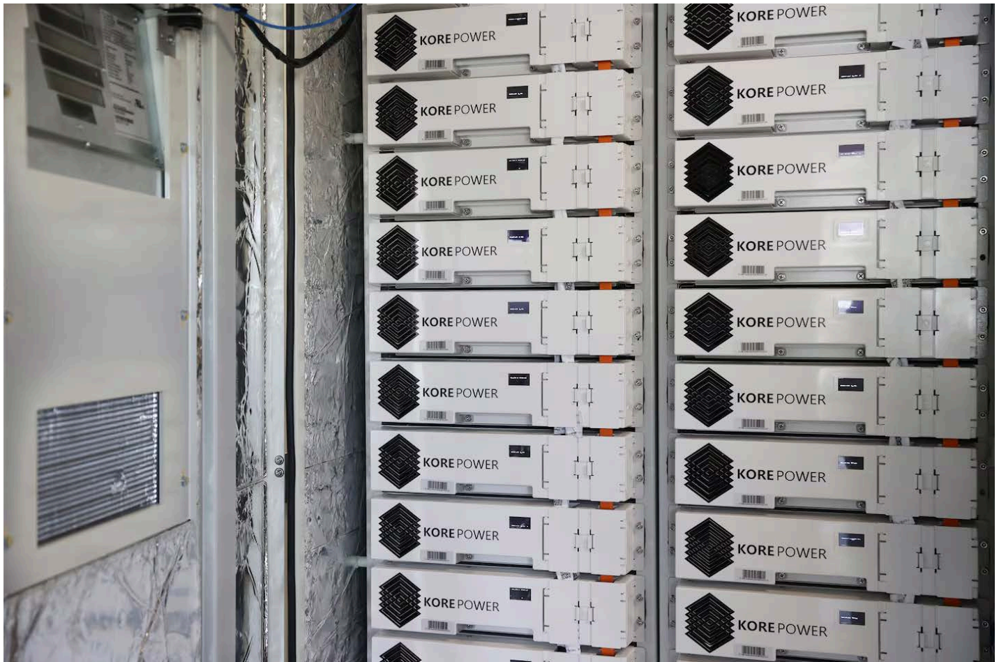
A close-up of the emergency battery system, which draws from solar energy generated on the roof to power the building in the event of an outage. JONATHAN WIGGS/GLOBE STAFF
