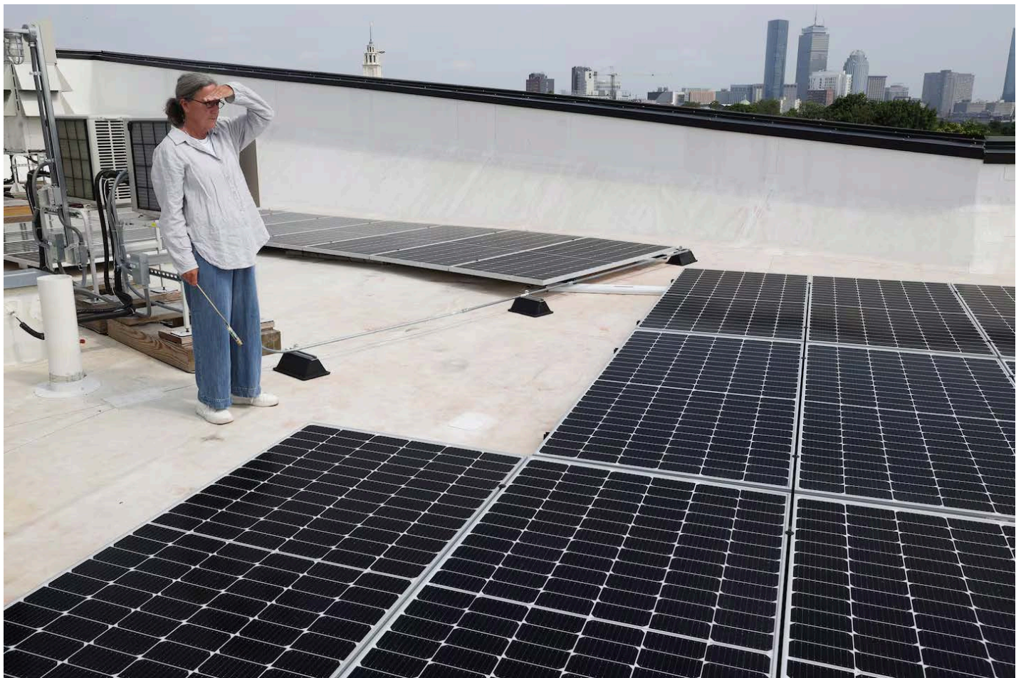
Building owner Julie Klump, with the Preservation of Affordable Housing, looks out over solar panels on the roof of The Kenzi at Bartlett Station, Boston's first fossil-fuel-free mid-rise apartment. JONATHAN WIGGS/GLOBE STAFF
